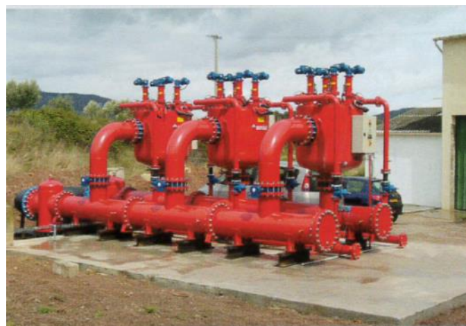
Picture 2 – Example of pressurised filtration system in Southern France
