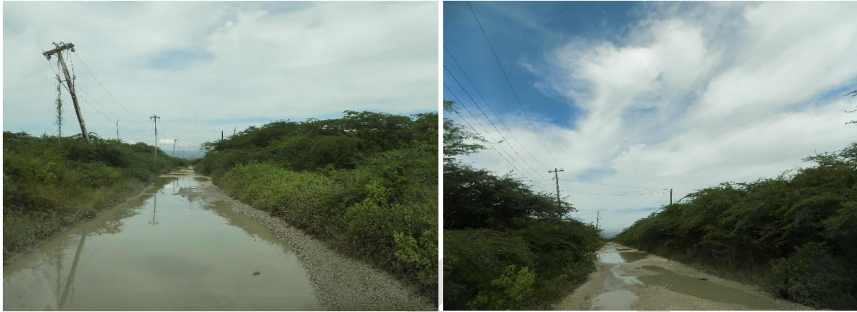
Figure 6.16: Flooded Road in Hill Run
