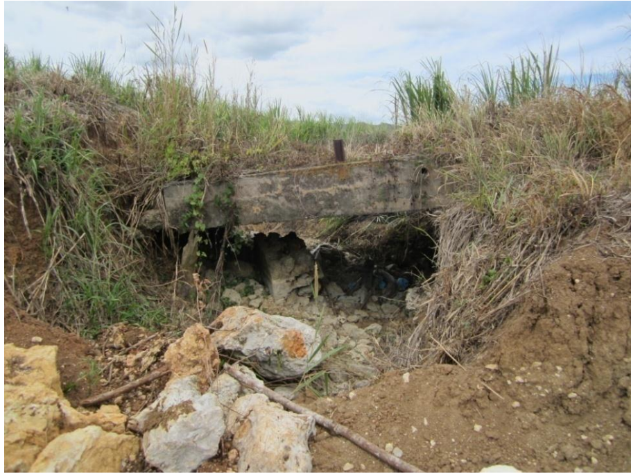
Plate 4.16 - A section of the Springvale river blocked by rubble.
