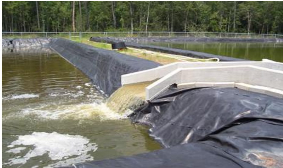
Plate 9.3 - Detention ponds used to reduce peak flows
