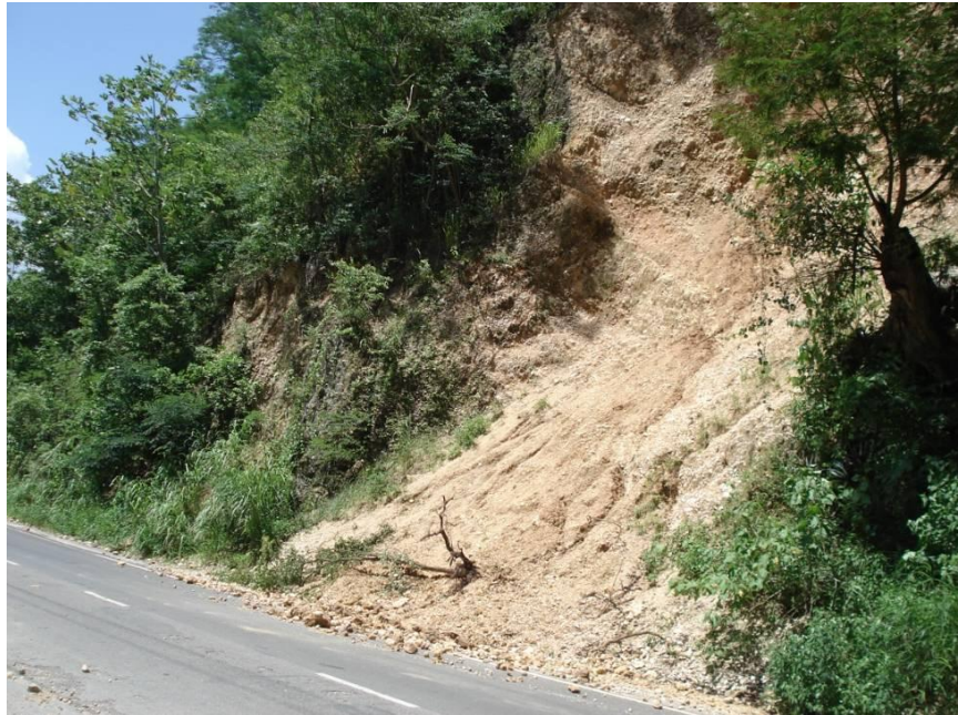
Plate 4.18 - Land slip on the southern edge of the fault zone exposed along the main road at the northern entrance to the Bog Walk Gorge (Walderston formation). This location is within the same Bog Walk Fault zone as will be traversed by the proposed highway.
