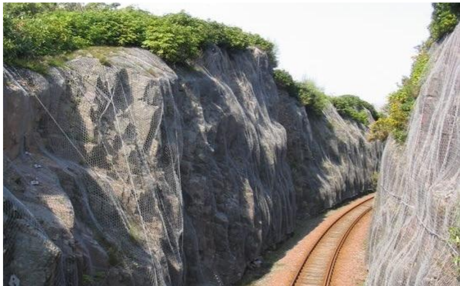
Plate 9.9 - Rockfall netting used to protect trains from falling rocks
