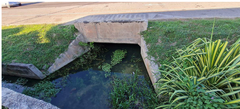
Figure 4-17 4.5x2m culvert from Gas Station to the channel west of The Peninsula
