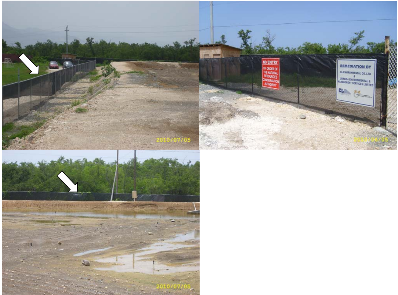
Plate 1 Photos depicting chain link fence with signage and shade cloth around the Landfarm
