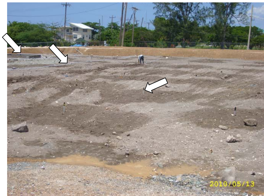
Plate 2 Photo showing irrigation pipes and sprinklers
