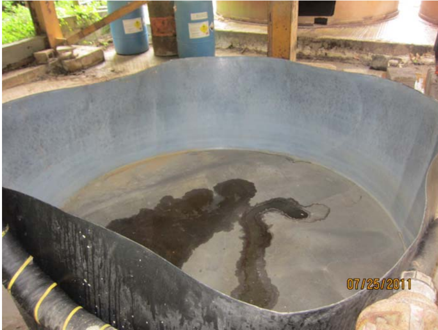
Plate 4 Photo showing leak/drip container
