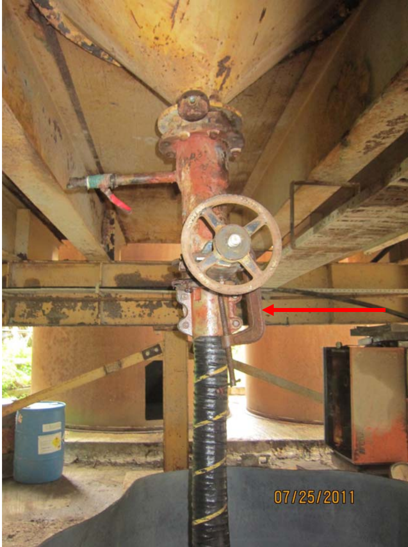
Plate 6 Photo showing “G” Clamp on valve
